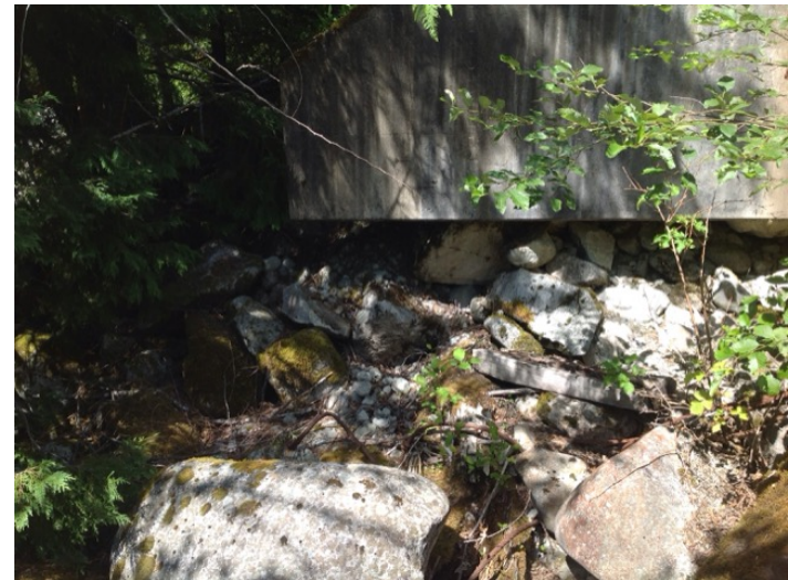
fill erosion from under the downstream right ballast wall
